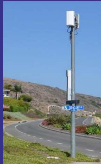
Small Cell Facilities – support 50' or less
